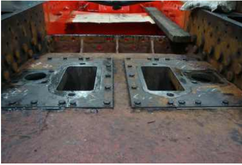
Blastpipe in 2 pieces have been finished and fitted. Mating faces for the blastpipe and main steam pipe have been faced up.
