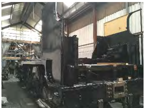
Frames and cab sides have been prepped and painted - all looking good.
